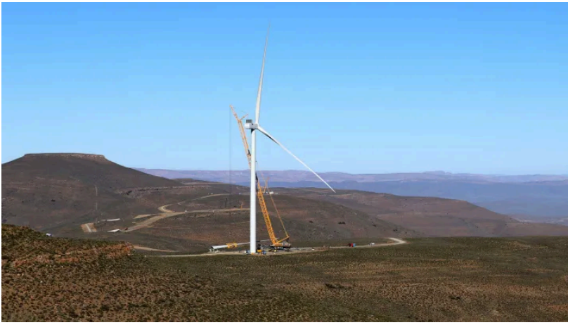
A wind turbine under construction at the Brandvalley Wind Farm. (Photo: Tamsin Metelerkamp)
