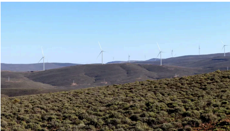
The Brandvalley Wind Farm under construction at a site along the boundaries between the Western Cape and Northern Cape. (Photo: Tamsin Metelerkamp)
