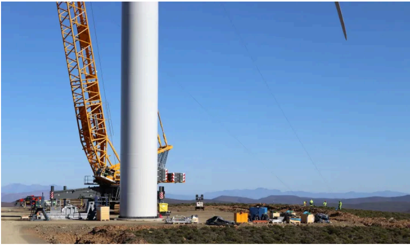
Workers around the base of a wind turbine under construction at the Brandvalley Wind Farm. The workers on the right are using long lines to adjust the angle of a blade being raised by crane. (Photo: Tamsin Metelerkamp)
